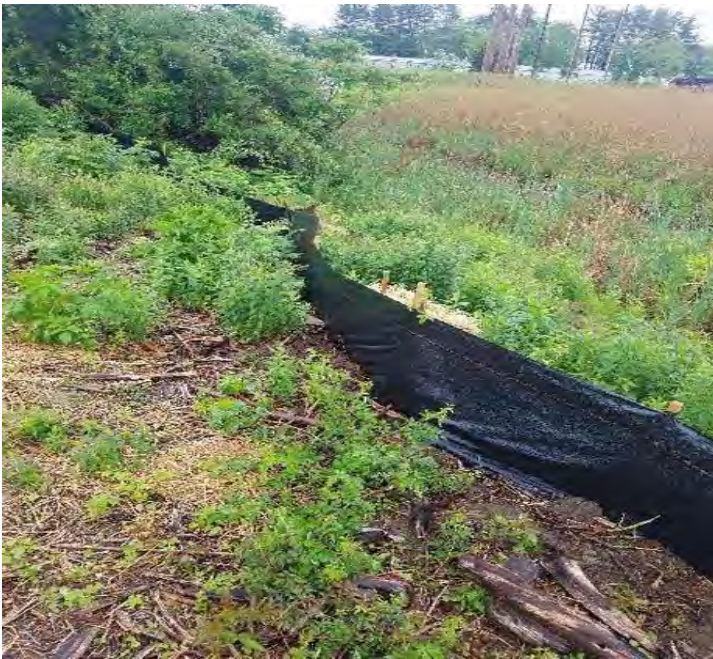
Fig 11: Silt fence installed between Str. F107-137 and wetland NM37, no maintenance needed. Viewing east. (6-11-19).
