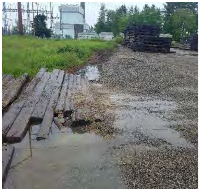
Fig 8: Combined berm installed around lay down yard, notice the water Runoff underneath the matting. Viewing north. (6-11-19).
