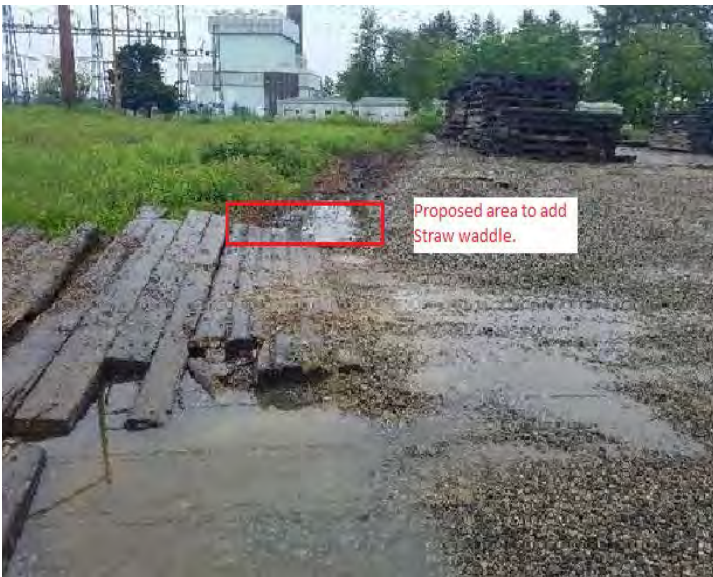
Fig 9: Proposed area in lay down yard to add straw bales, this would help filter The runoff water that channels under the timber matting. Viewing north. (6-11-19).
