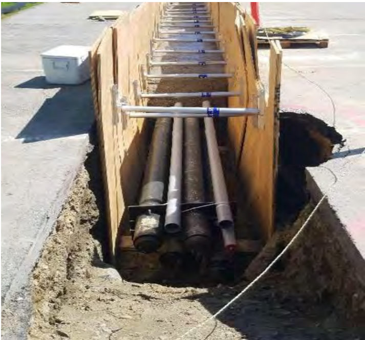
Fig 15: McCourt began to pour concrete duct bank over installed pipe in A lot. Viewing south. (6-12-19)
