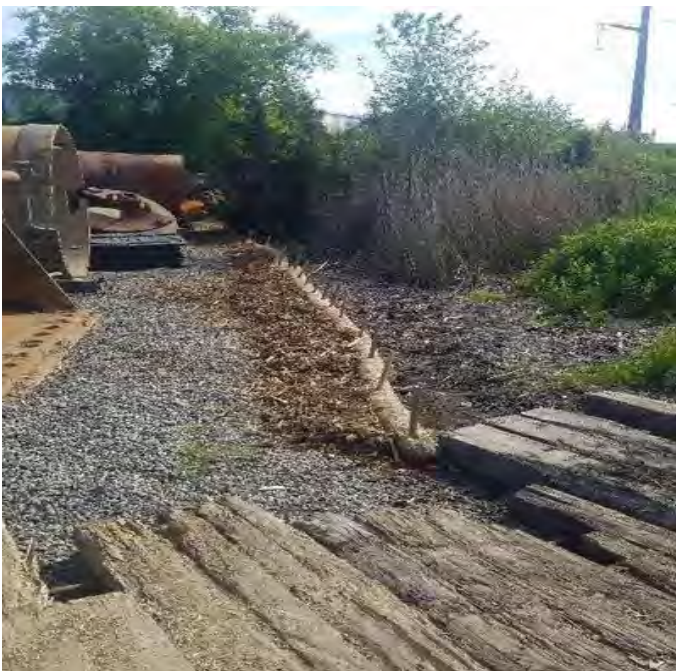
Fig 3: Combined berm installed around lay down area off of Gosling Rd. Viewing south. (6-10-19).
