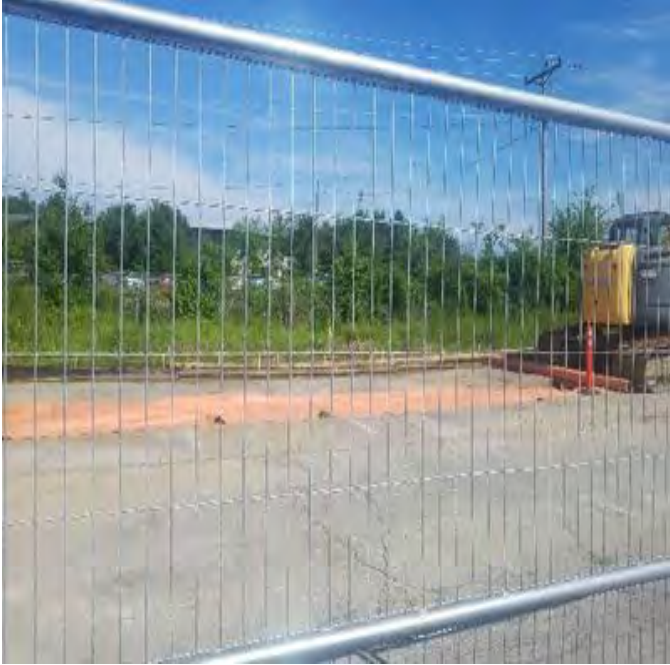
Fig 1: McCourt continues to trench and assemble duct bank in A lot. They laid filter fabric over the exposed trench to prevent water from running through. Viewing southeast. (6-10-19)
