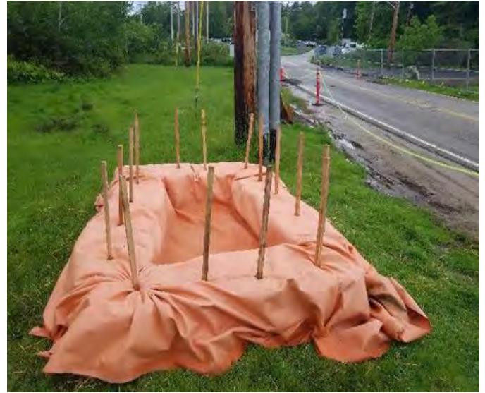
Fig 14: The dewatering discharge basin next to Colovos Rd. The BMP structure will need to be expanded to encase the filter bag. Viewing south. (6-11-19).
