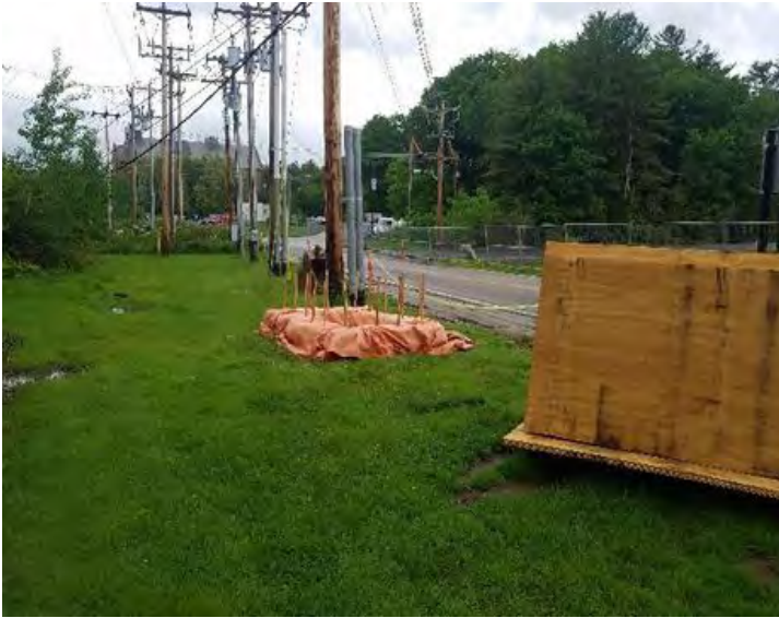
Fig 13: The dewatering discharge BMP basin the McCourt installed for the trench dewatering activities next to Colovos Rd. Viewing south. (6-11-19).
