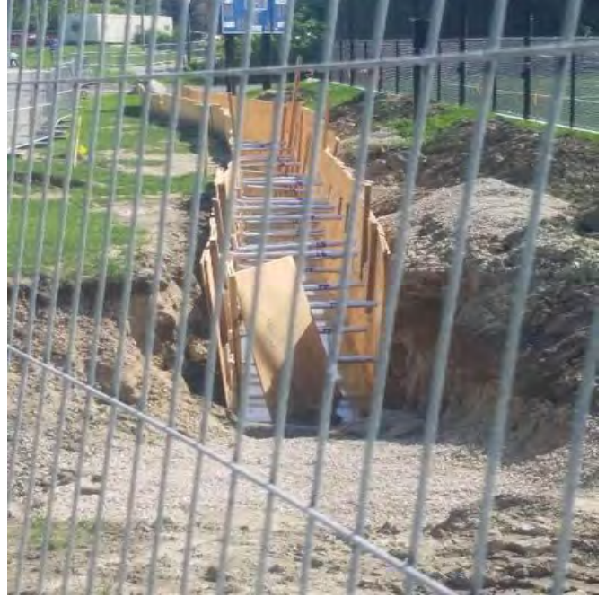
Fig 2: Water is still present in the trench near the rain garden, along Colovos Rd. Viewing south. (6-10-19).
