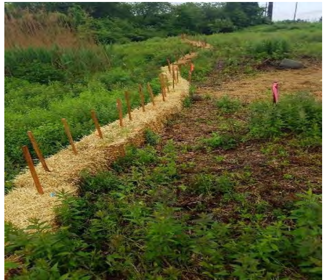
Fig 10: Straw bales installed correctly between Str. F107-139 and wetland NW37. Viewing north. (6-11-19).
