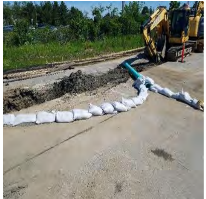
Fig 16: McCourt's temporary water diversion plan; diverting water run off over their trench. Located in the low area in A lot. Viewing southeast. (6-12-19)
